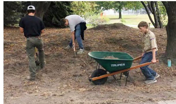
Members of Boy Scout Troop 110 helped backfill the edges of the newly finished paved walking trail around the Franklin-Cotterell Greens in North Bend. FACF recently provided a $30,000 grant to help finish the decades-long project.
